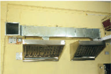
Wall Mounted Hood with Ductline
