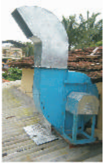
Blower Machine with Chimney
