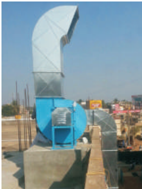
Blower Machine with Chimney
