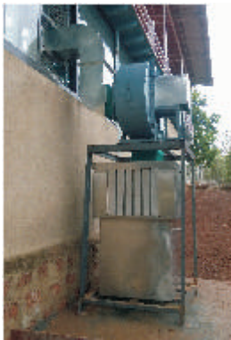
Water tank Filtration Systems
